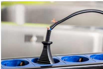
Use of bare cables
