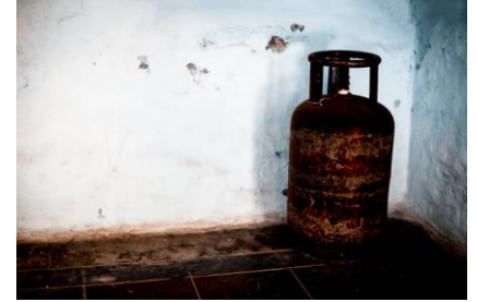
Improper storage of gas cylinder
